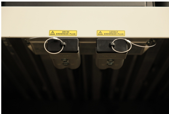
JUMPSTART RECEPTACLE (TRUCK) Crank battery
